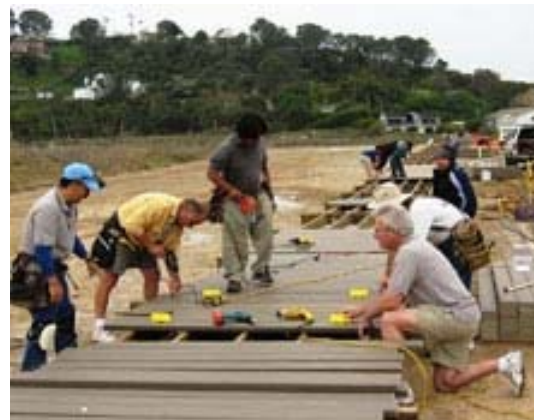
Members from the Rotary Club of Del Mar, California, USA, give a helping hand on the construction of a new boardwalk that will run through the San Dieguito River Park.
